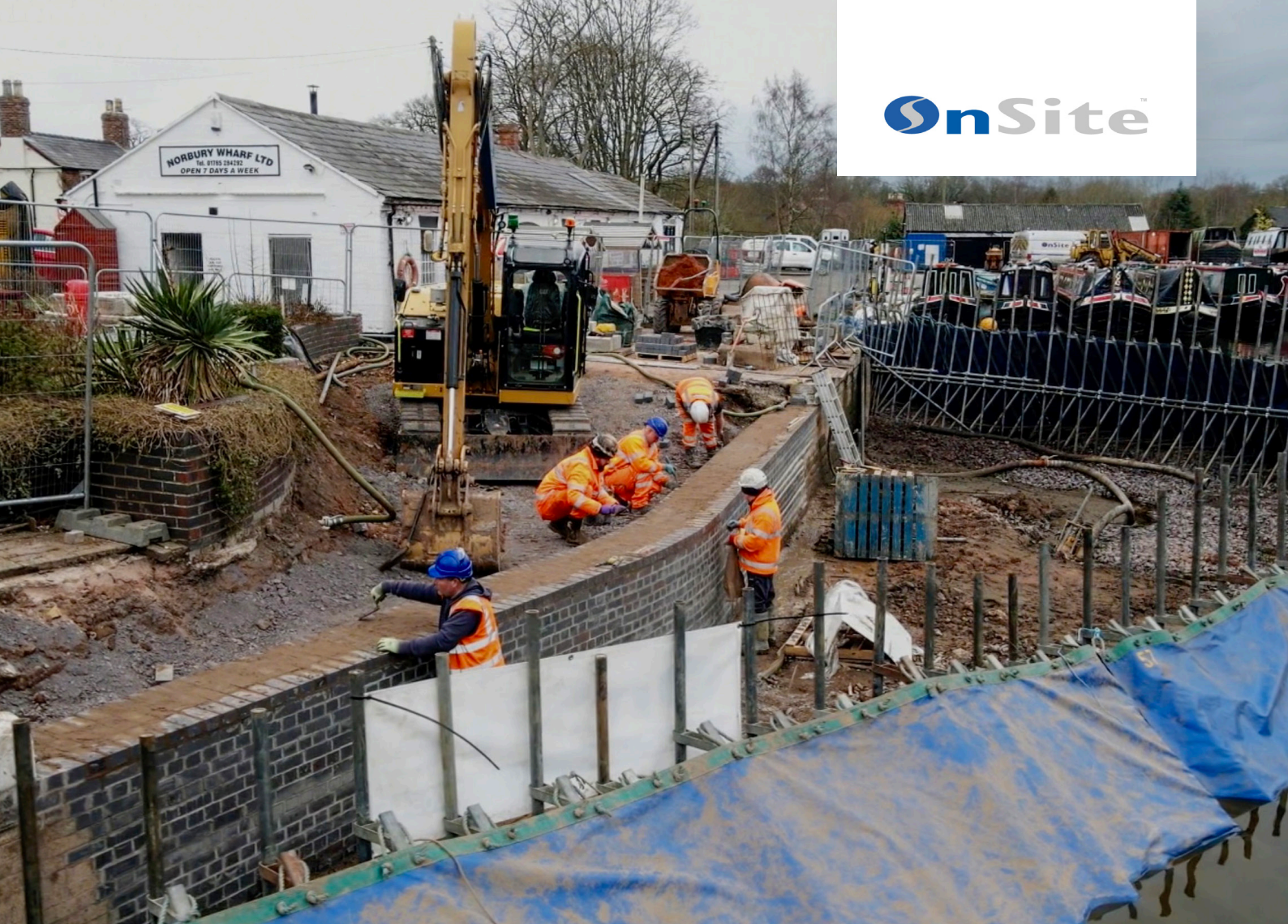
Workers rebuilding the new brick built wall behind the protection of PortaDam.
